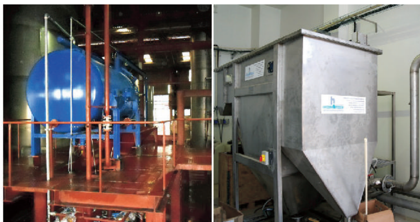
Figure 4. Different industrial wastewater treatment technologies can be applied in the same industrial sector. This example from the vegetable oil industries where a closed-circuit water cooling system (photo to the left) and chemical and physical treatment (photo to the right) were adopted as needed
